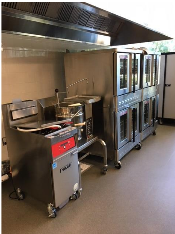
Front Wall Equipment
