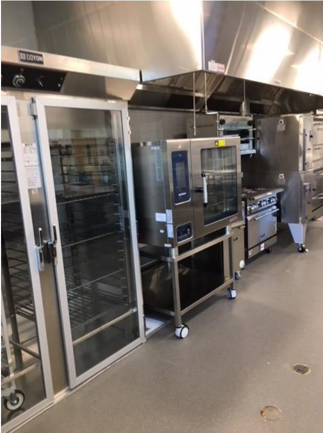
Back Wall Equipment
