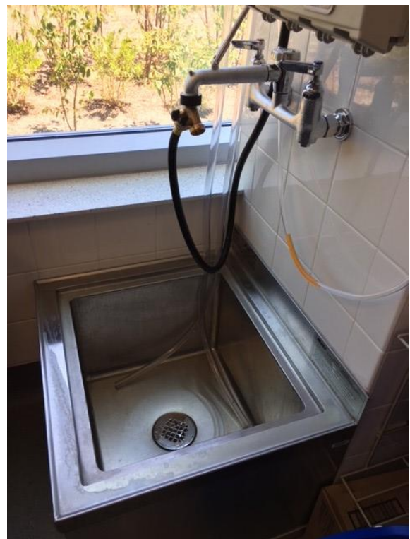
SanRoom Water Access
